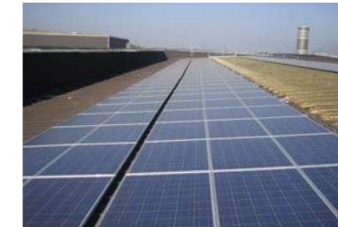
Quadrifoglio S.p.A., 296 kW for a composting plant, Florence
