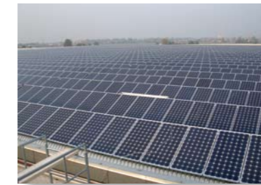
Comet S.p.A., 1 MW PV system roof-mounted on the megastore, Bologna
