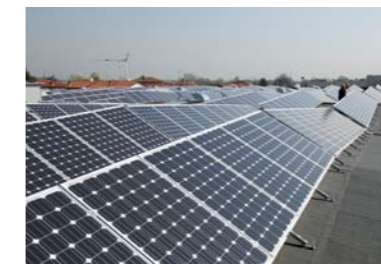
Endress + Hauser Sicestherm, 192 kW PV system on industrial building, Milan
